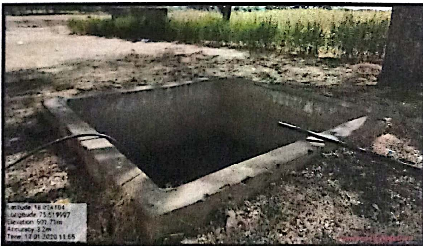
TANK FOR WATER STORAGE
